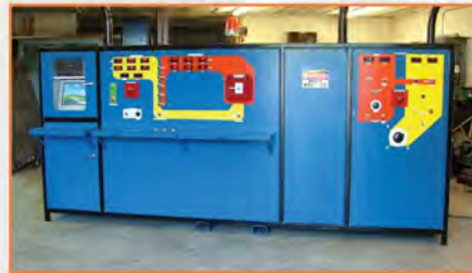
Our 750 KVA Test Panel handles 230/460/575 and 2300/4160 volts
